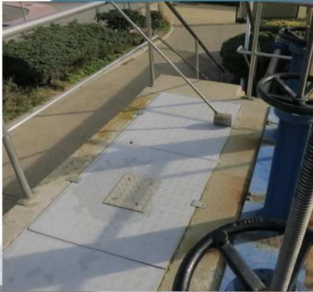
Biological treatment inlet
